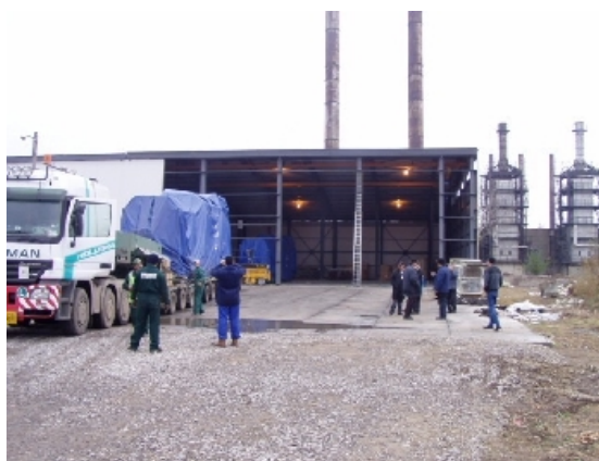
Arrival of a combined heat and power plant for bearings manufacturer Rulmenti Barlad. UNDP GEF financed the Feasibility Study for this 17.5 million energy efficiency investment.
